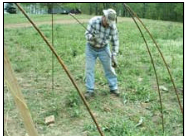
Figure 26 - While the tripod is holding the dome, place the Parallel Arcs inside the Ground Circle and fasten them with stainless steel U-bolts on the 26 1/2'' marks provided earlier.
