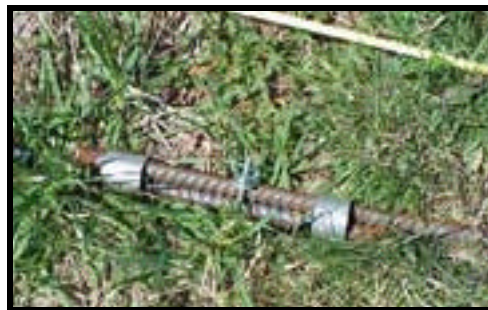
Figure 16 - Ground Ring Connection
