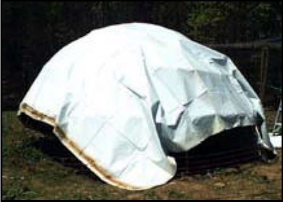
Figure 50 - Drape a 15' wide X 25' long piece over the center as pictured and cut and tuck prior to fastening to the Middle Circle. The door is to the far left in this picture.
